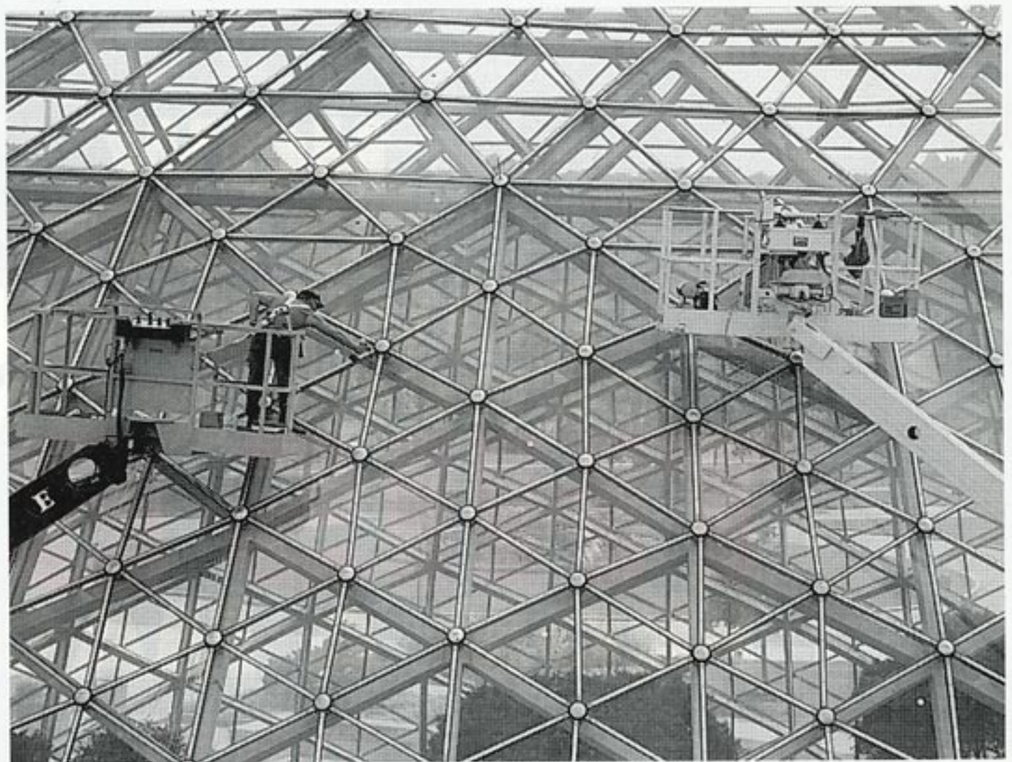
Working as high as 80-feet above the ground, Choice Construction employees wear body harnesses to keep them secure when working on the lifts.
