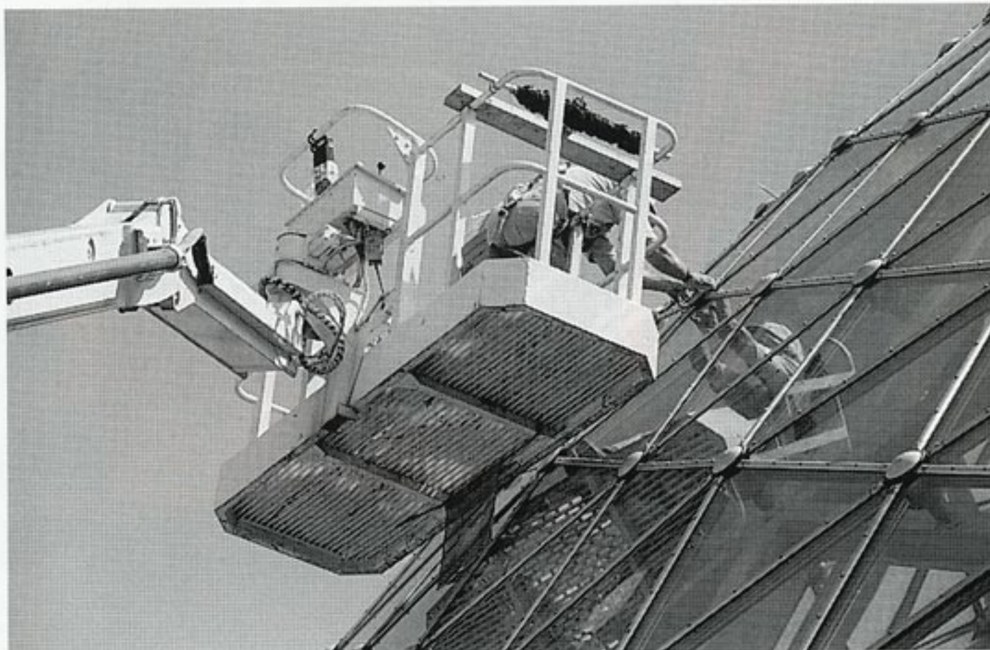
All hub covers, hub cover gaskets, and gaskets around and under aluminum frames, as well as 97 glass panes are being replaced in the job this summer and early fall at the Show Dome.
