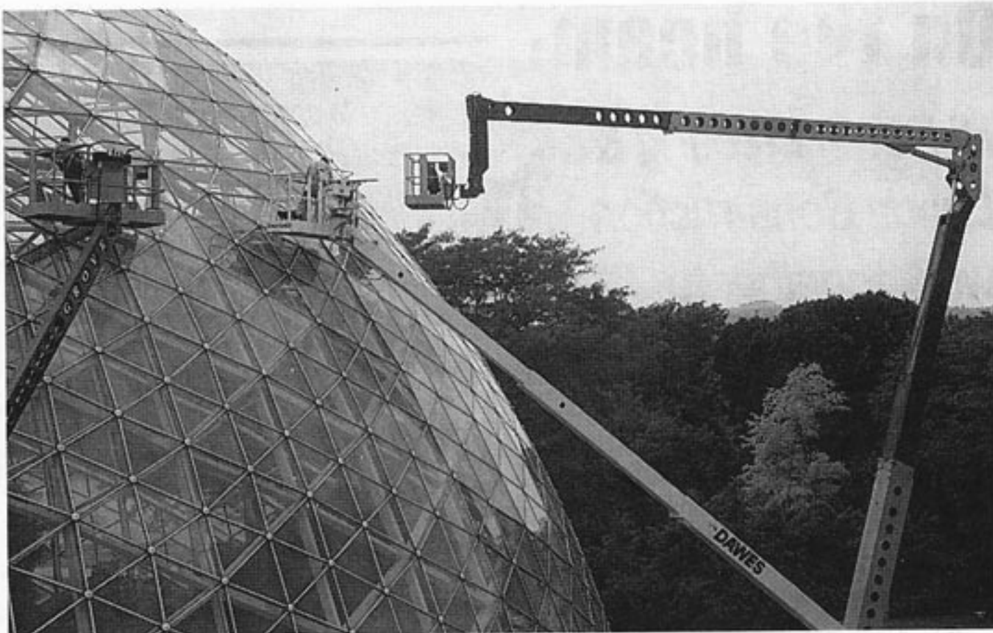
Choice Construction employees in lifts work on one triangular section at a time, and then move the lift before starting on the next triangular section of the dome.
